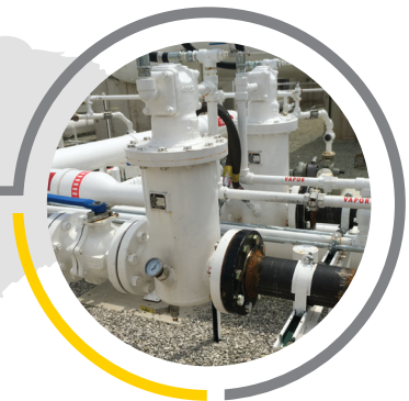
Flow Components Strainer and Air / Vapor Eliminator
